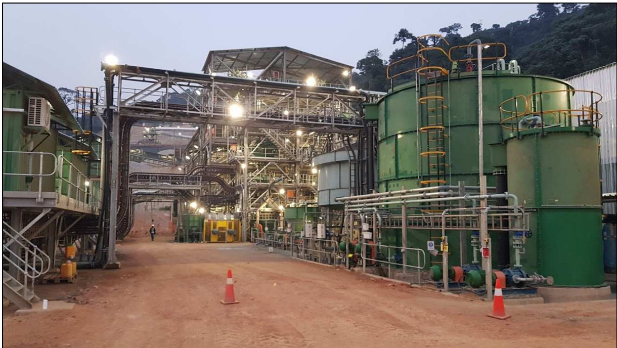
Gravity recovery plant
